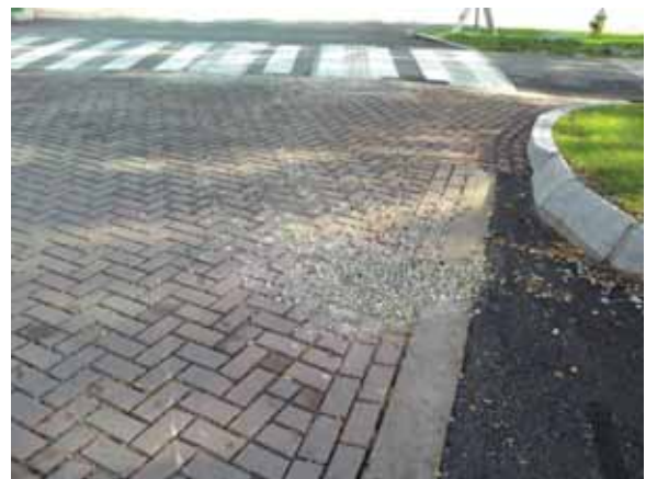
Figure 17: Run on from intersecting MUB drive.
