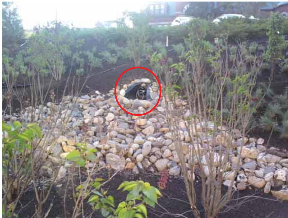
Figure 6: Picture of T Lot effluent location. T Lot is to the upper right in this picture.
