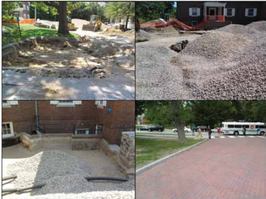
Figure 1: August 2010 installation of PICP system (clockwise from top left) demolition and excavation, placement of subbase aggregate, finished product, underdrain installation.
