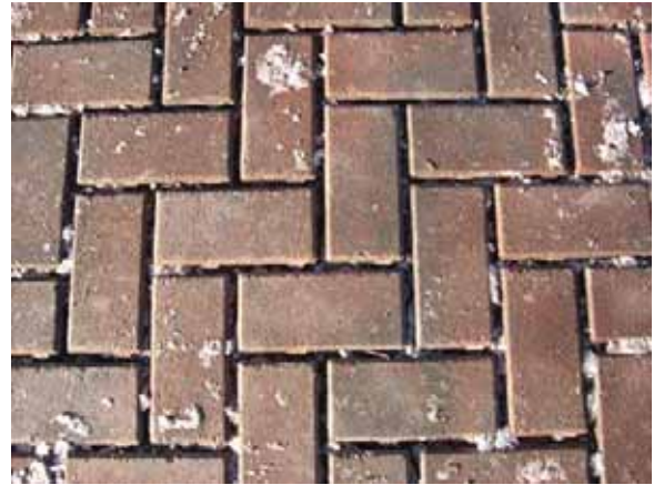
Figure 15: No. 8 joint stone has settled approximately 1 inch.
